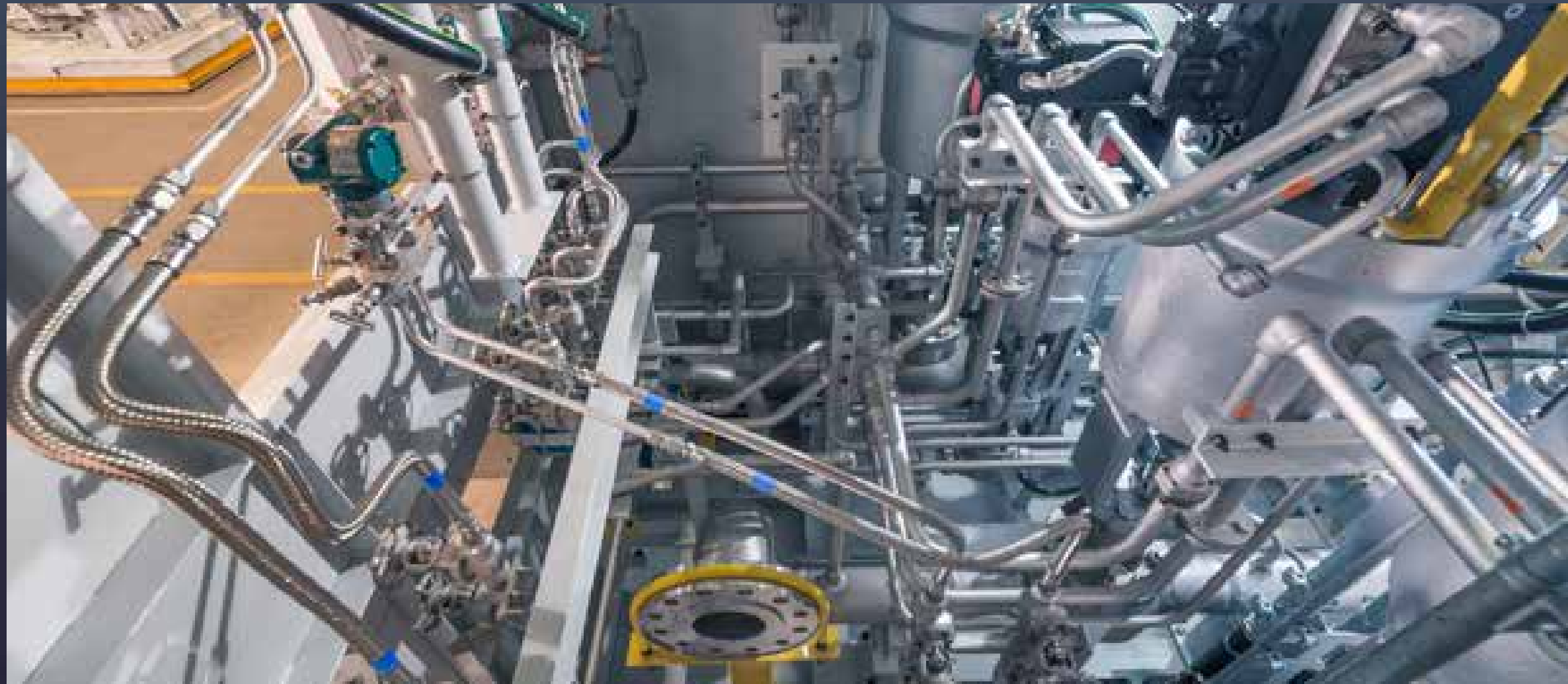
MITSUBISHI POWER M701 F4 FUEL GAS SKID
