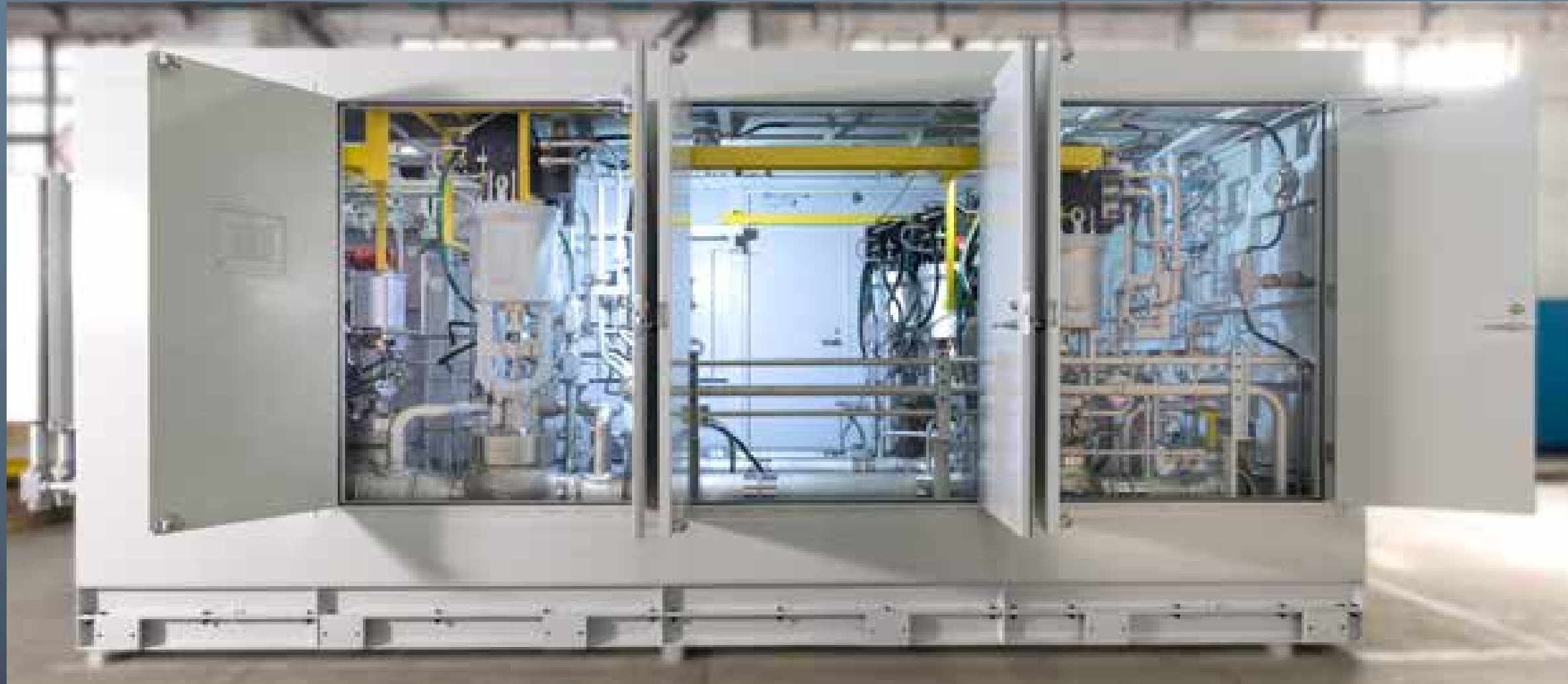
MITSUBISHI POWER M701 F4 FUEL GAS SKID
